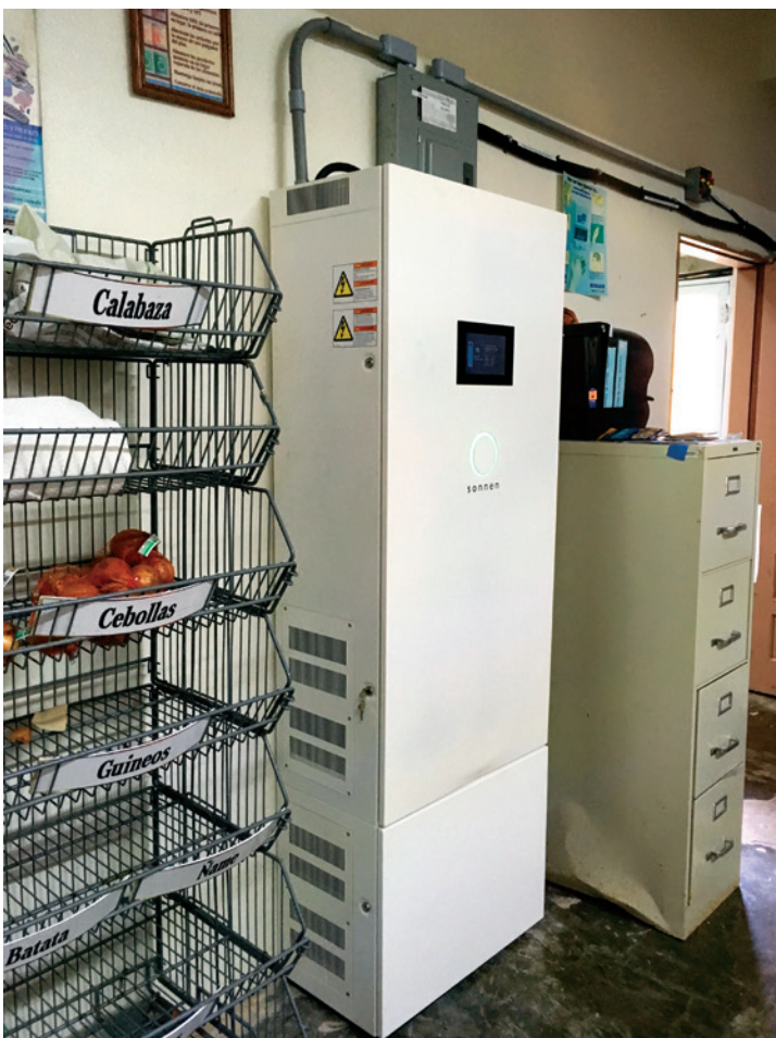
Residential and small commercial battery systems, like this 14-kilowatt-hour sonnen eco 14 battery at a remote school in Orcovis, Puerto Rico, tend to have an average installed cost between $1,000 to $1,400 per kilowatt-hour.
