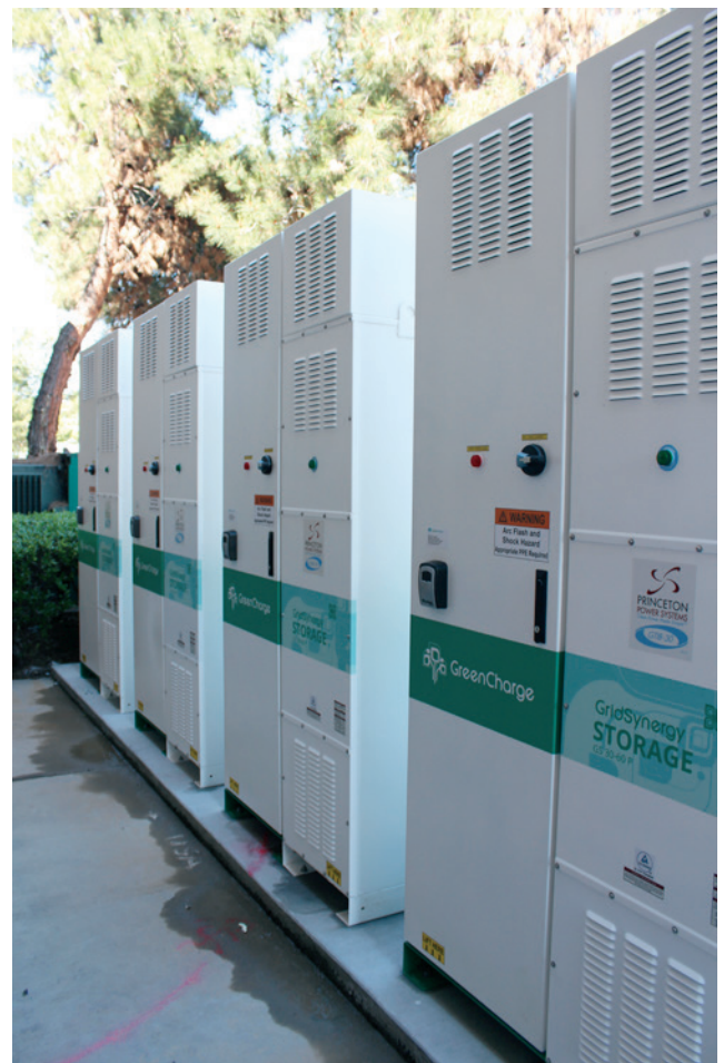
Battery systems in the 100 kilowatt-hour to 500 kilowatt-hour range, such as this system at a Safeway supermarket in San Jose, CA, typically cost less than smaller systems, around the $600 to $800 per kilowatt-hour range.
