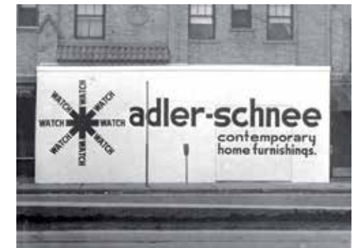
Adler-Schnee Livernois storefront under construction, Detroit, 1954. (Courtesy Cranbrook Archives, The Edward and Ruth Adler Schnee Papers.)
